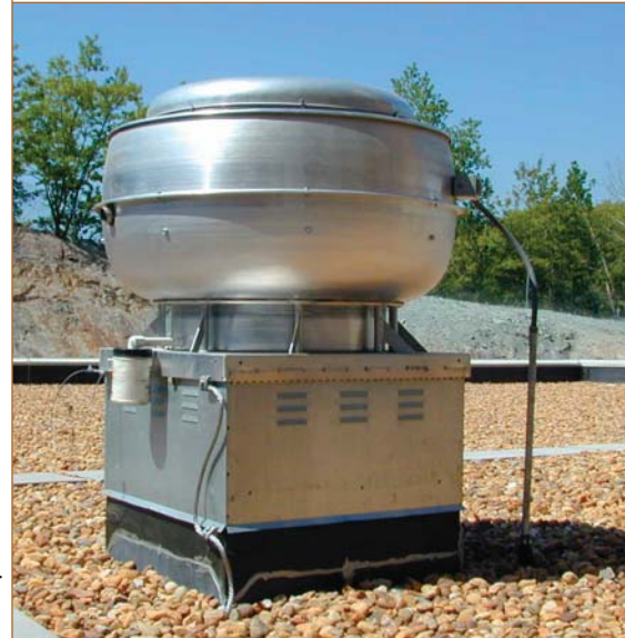
Roof fans and exhaust ducts are covered by NFPA 96.
